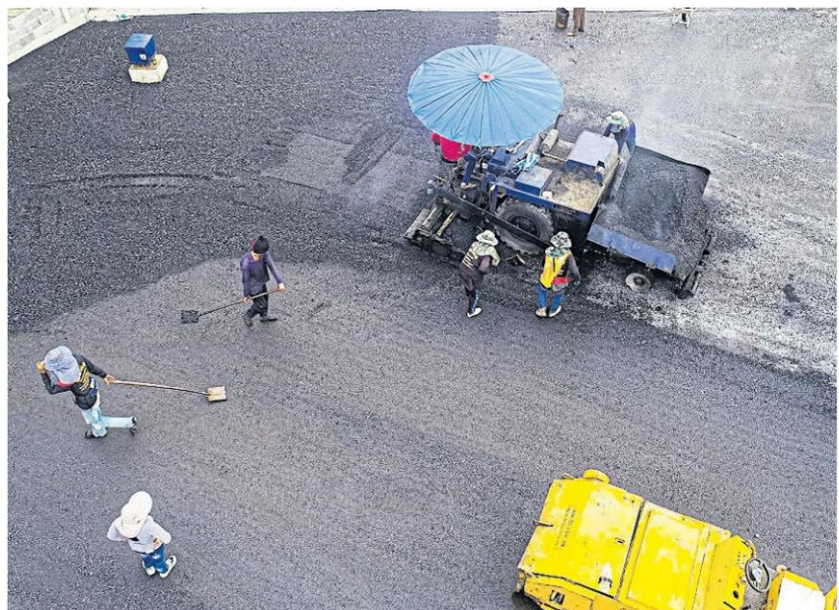
Workers pave a road with asphalt made from plastic waste which will help promote effective waste management. PHOTOS BY DEPARTMENT OF HIGHWAYS
